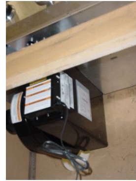
Vent Fan Housing Rating Plate
